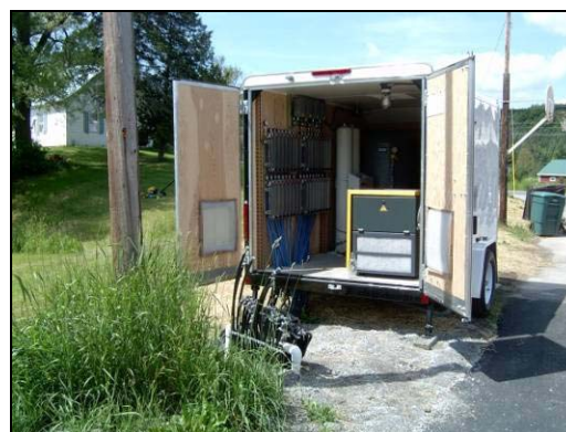
Figure 3. Oxygen Injection System
