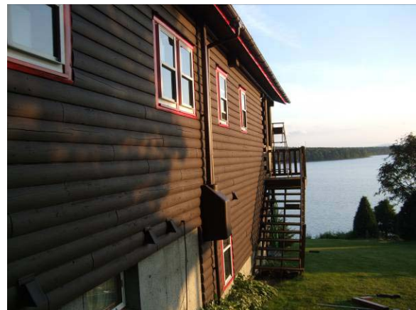
Figure 3. Radon system after final installation
