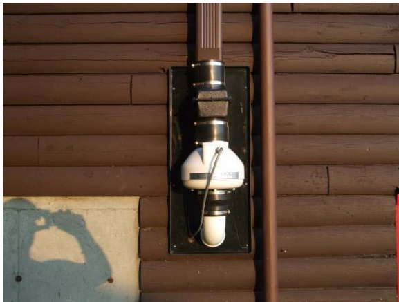
Figure 1. Radon system with fan mounted on the exterior of the house
